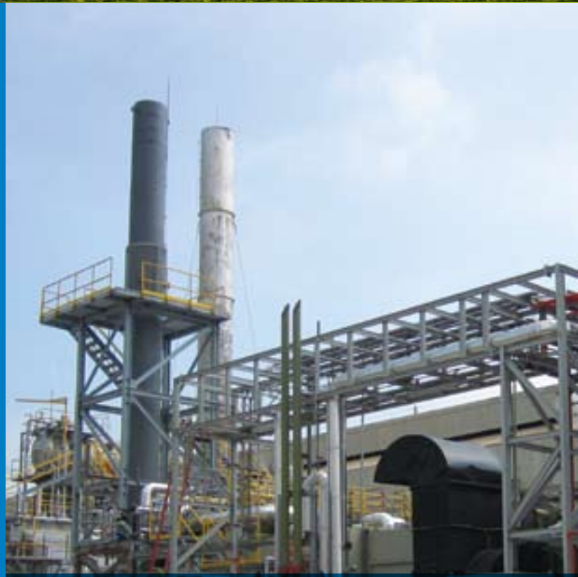
To optimise the energy situation at the Smurfit Kappa Barranquilla mill in Colombia, a new CHP installation has been installed.
